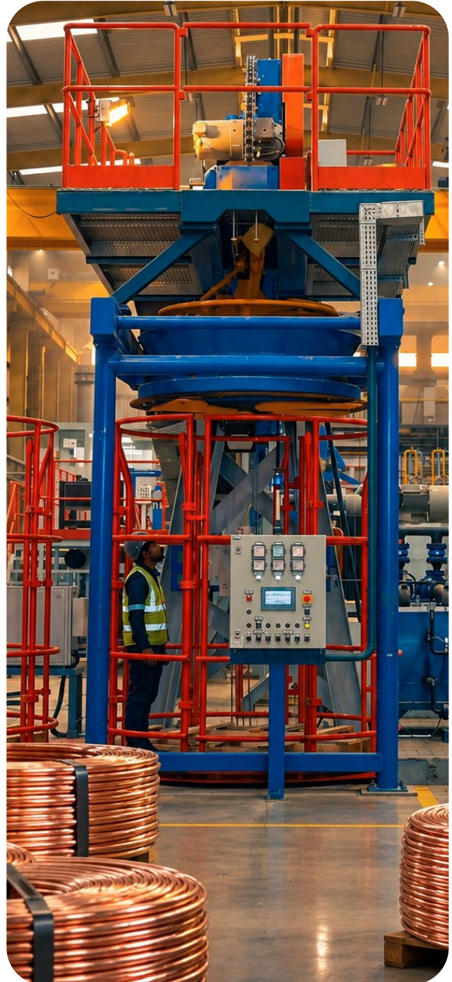
02 Coiling stations in the production hall
